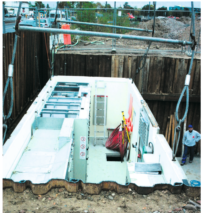
Saves space and is not visible: The traction power substation in the underground concrete container
