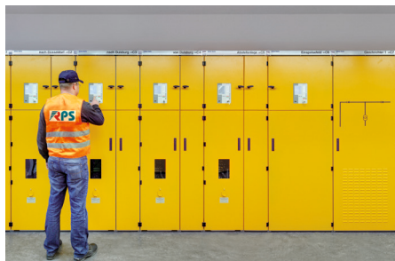
Switchgear panel – assembled as needed
