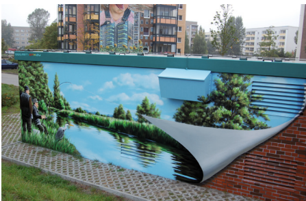
Turnkey substations – here for ViP Potsdam
