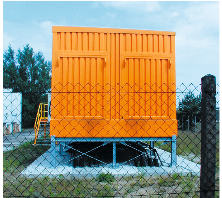
Substation in factory-made steel container – e.g. for Vattenfall (DC 2.4 kV)
