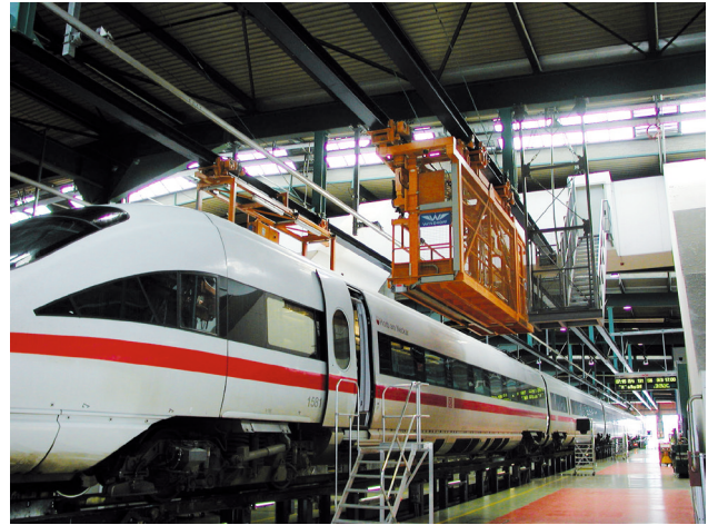
Depot – here in the ICE works at Frankfurt-Griesheim with multi-voltage supply switchgear panel
