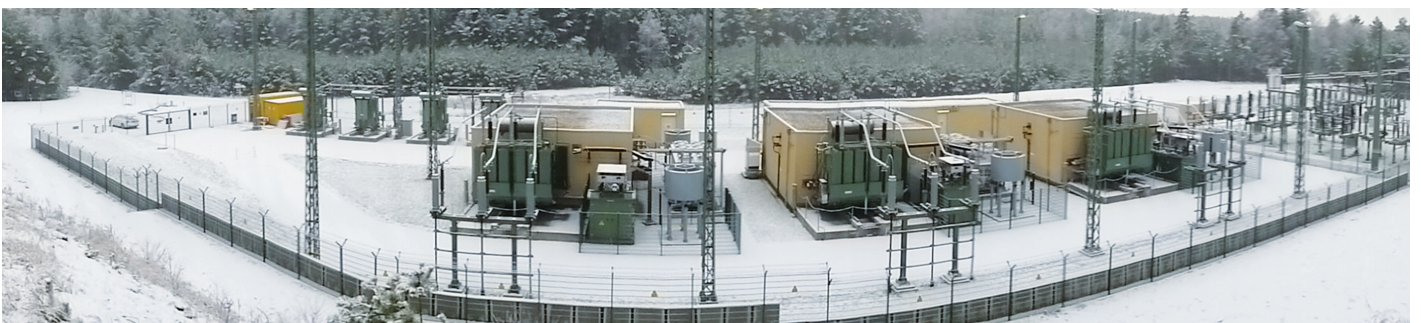
The inverter station of DB Energie Lohsa-West
