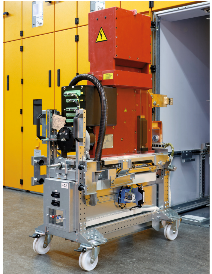
Circuit breaker truck with GE Gerapid DC high speed circuit breaker
