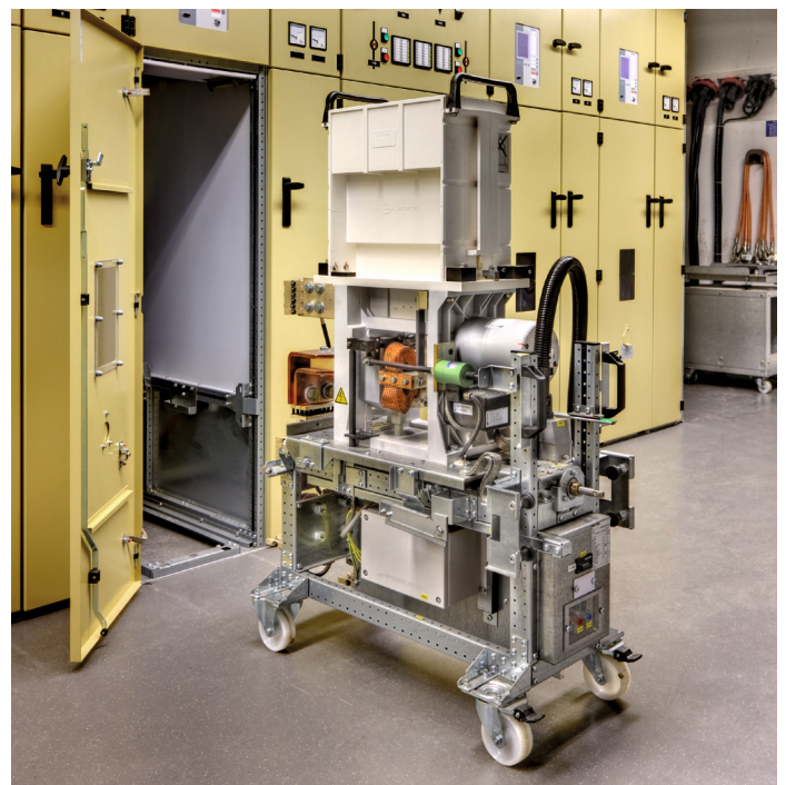
Circuit breaker truck with Sécheron UR DC high speed circuit breaker
