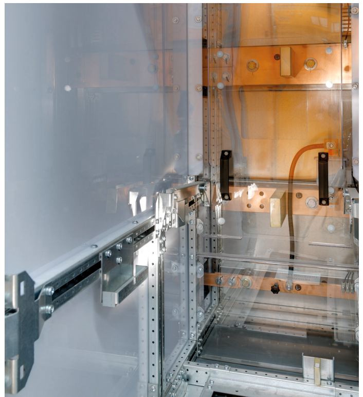
View of the circuit breaker panel – power compartment in the foreground, behind: the shutter of the busbar and cable connection compartment
