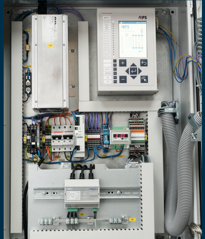
Interior view of the TracFeed® RCM monitoring system control cabinet
