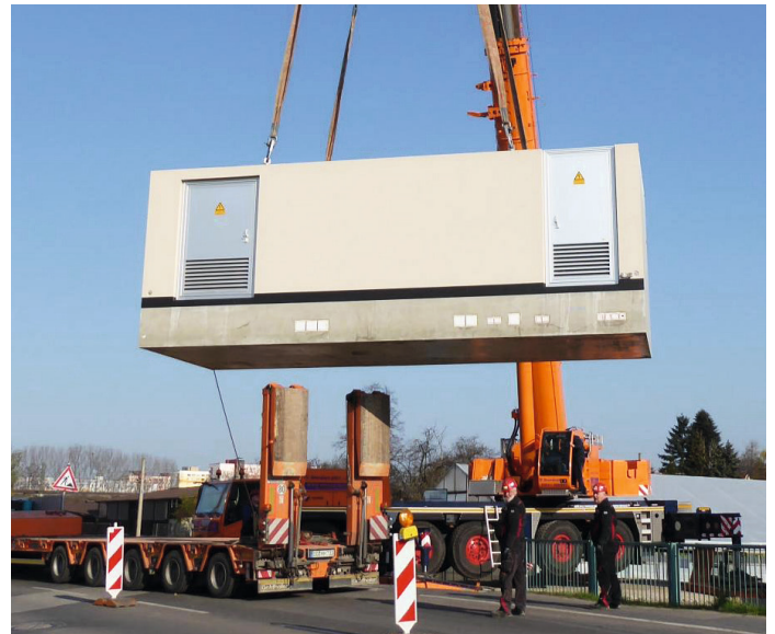
Concrete version of the KGUW being lifted by crane off the transporter
