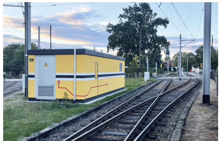
KGUW positioned in a terminal loop at the final installation site with short cable paths
