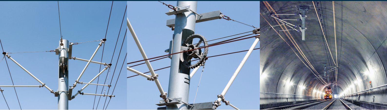
Assembly Stuttgart Zuffenhausen - TracFeed® ALU 1000
