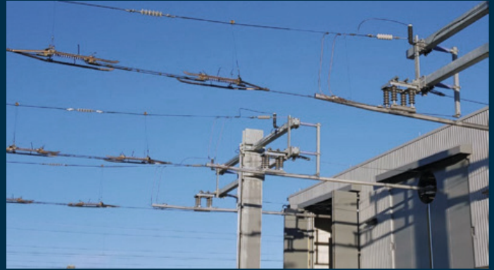
Section insulator arrangement in Denver/USA
